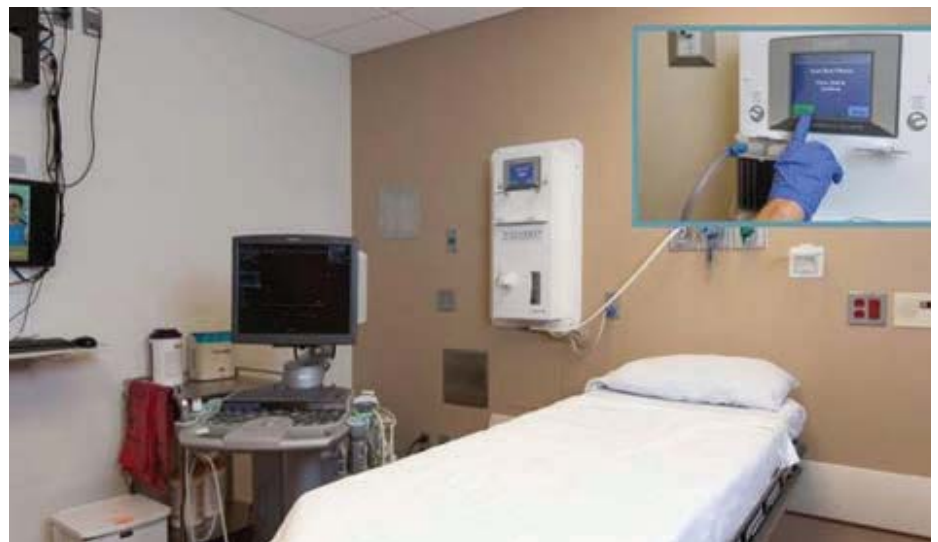
Figure 1 • The New System Set Up
